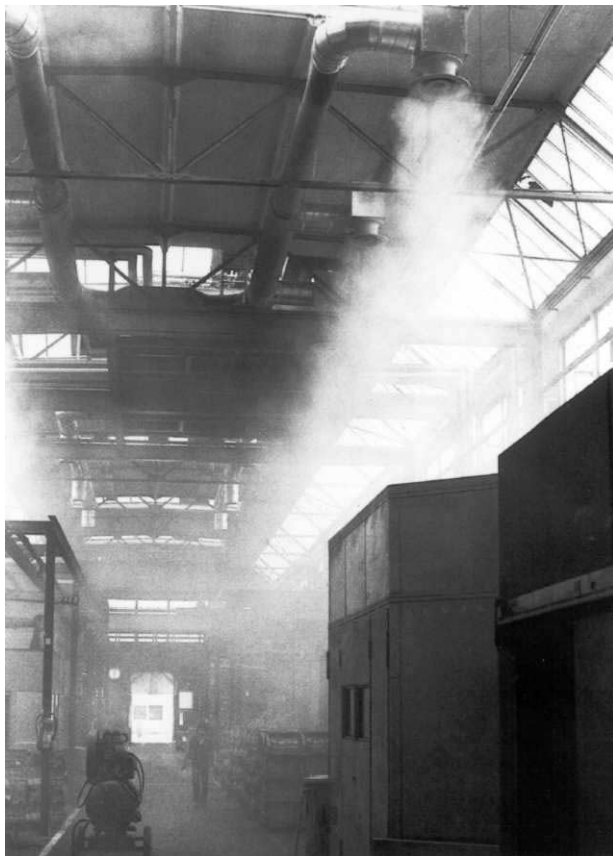
Jet spread in heating mode made visible with smoke tracer: The warm, vertical supply air jets penetrate deep into the occupied zone.
